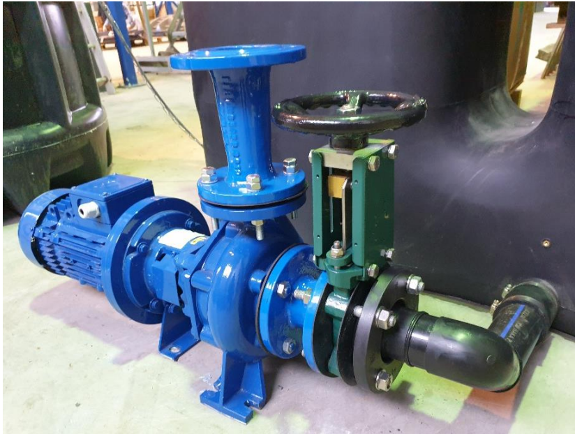
Figure 14. Fitting of Disposal Pump
